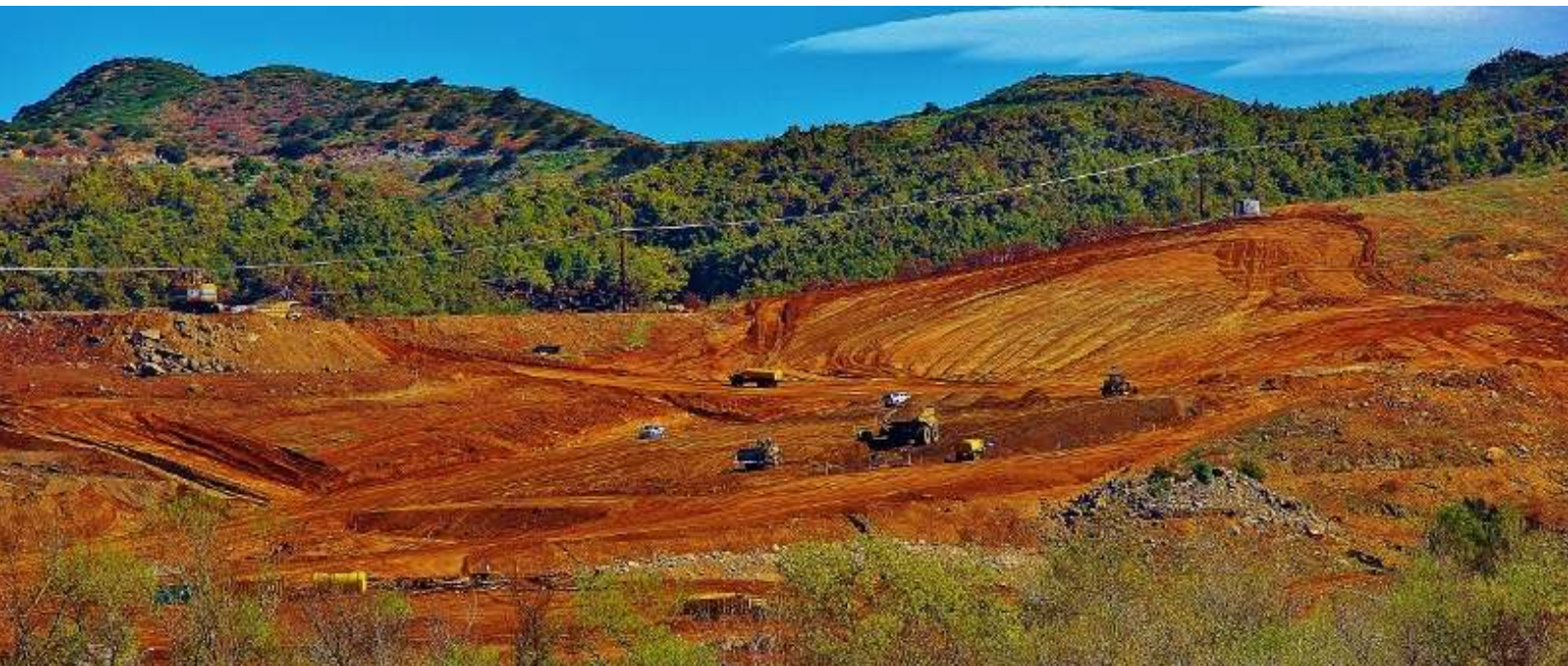
To the far right of our field, this construction is taking place for more homes!
