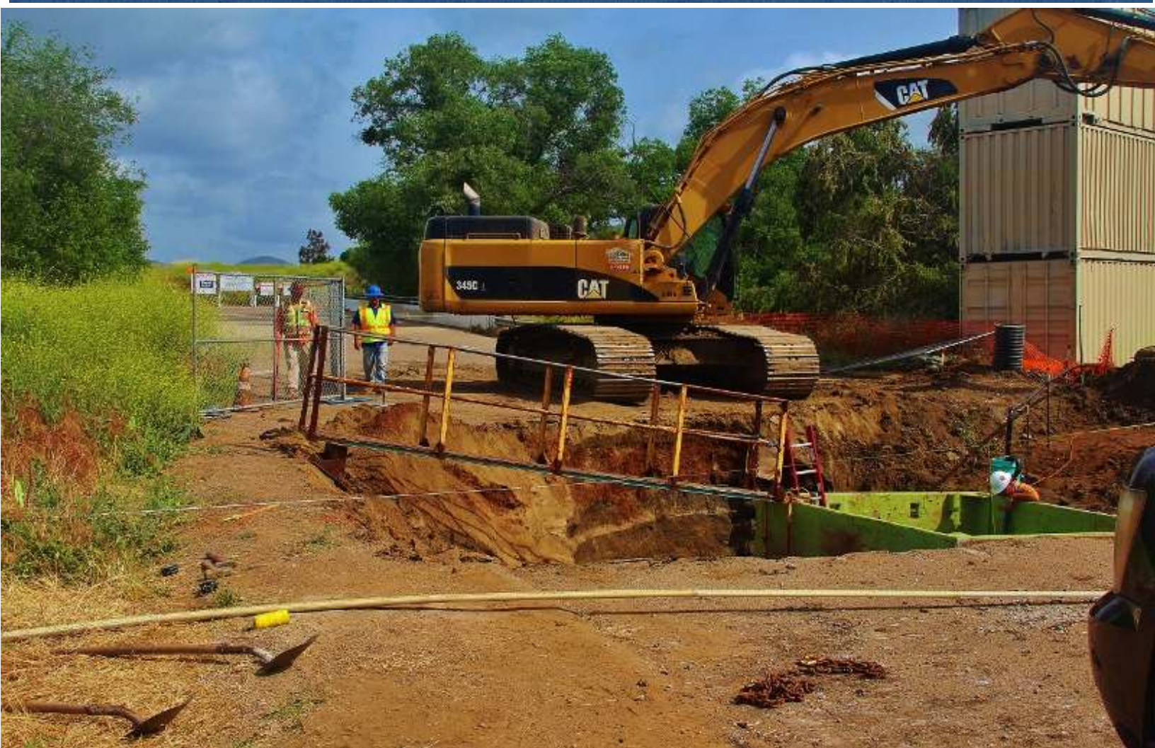
Here is the reason why we could not gain access to our field. This was taken just before the bridge in front of our main gate. The hole is about 20 feet deep and cuts across the entire road. 4/25/2017
