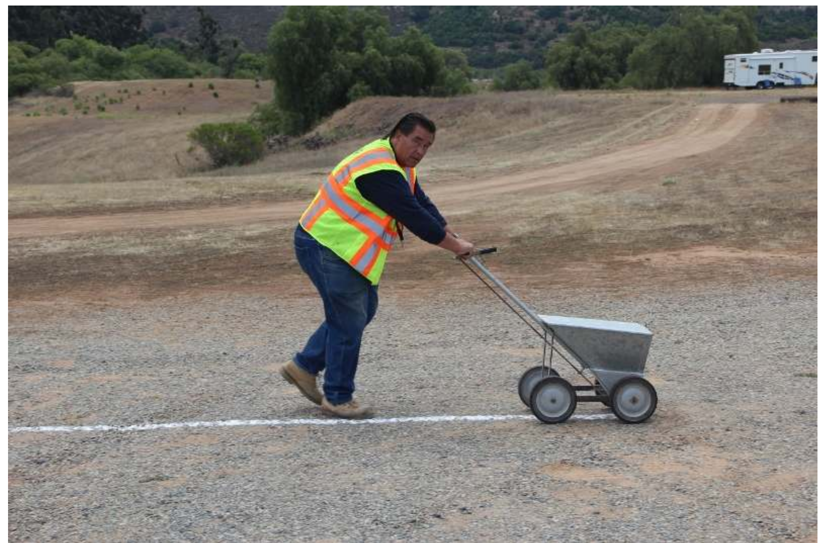
Safety Officer Jim Jenkins limed the areas that needed to be marked.
